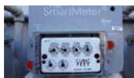
Automated Meter Reading
